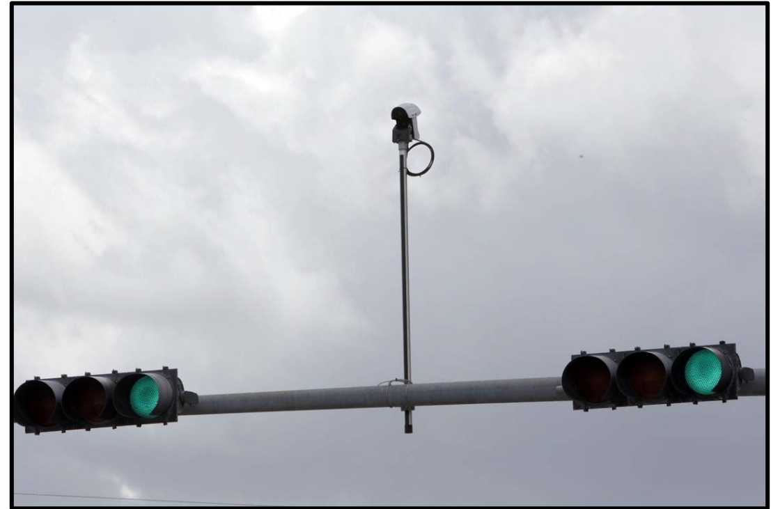
Vehicle detection upgrade at the signalized intersection of Lost Tree Village/Old Harbour Road
